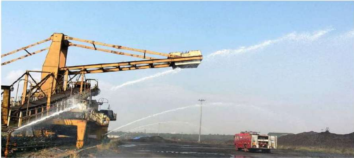
WATER SPRINKLERS AT COAL STACK YARD
